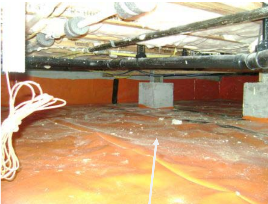
This example (not a photo of your house) has a ground vapor retardant barrier made from thick reinforced polyethylene. All joints are taped. The edges of the polyethylene are glued to the foundation wall and taped around pier blocks. There is also closed cell polyurethane foam insulation sprayed underneath the subfloor. This not only insulates the floor but creates a moisture and air barrier seal between your living space and the crawlspace, reducing infiltration. We are not recommending insulating your floor at this time because of your mild climate and the high cost of foam (about $4.00 per square foot at 3" thickness.)
