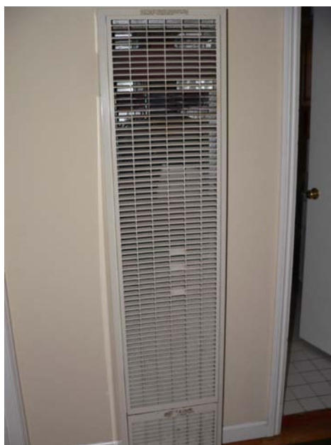
Williams wall furnace to be replaced.
