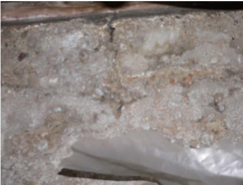
Foundation wall in old portion of house has voids, but no large cracks.
