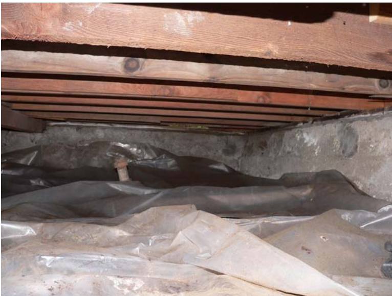
Polyethylene sheet in crawl space does not cover ground fully, is not sealed to foundation and will not withstand technicians working on it.
