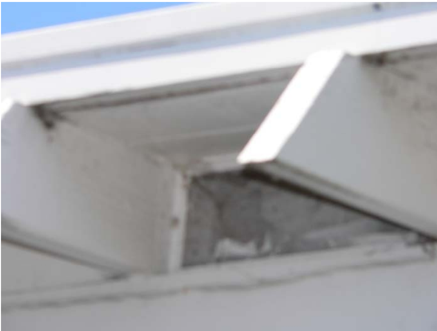
Looking for insulation in cottage attic from outside since attic hatch inside was inaccessible. Result inconclusive.
