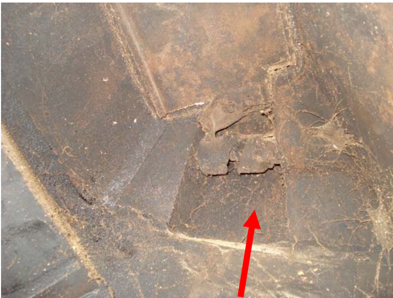
Damper in fireplace has large “holes” and was a significant source of air leakage.
