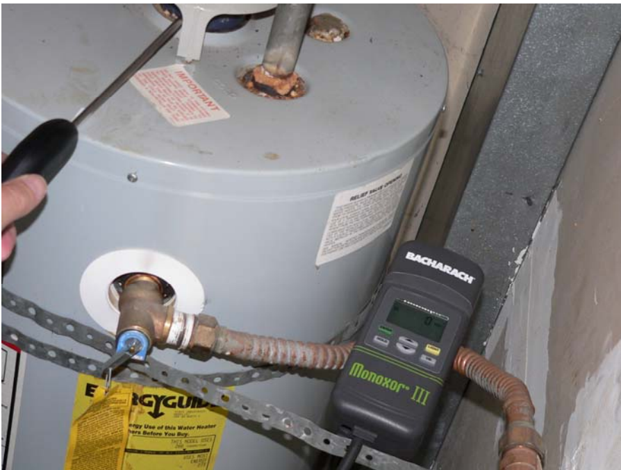
Measuring carbon monoxide content of cottage water heater flue gas. The reading was low, which is good.
