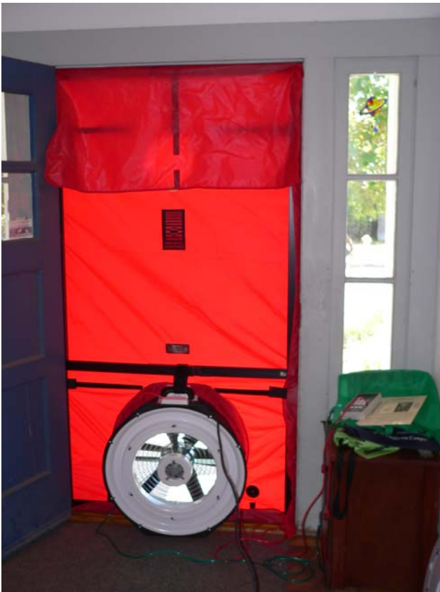
Blower door test in process. We noted a high level of envelope leakage.
