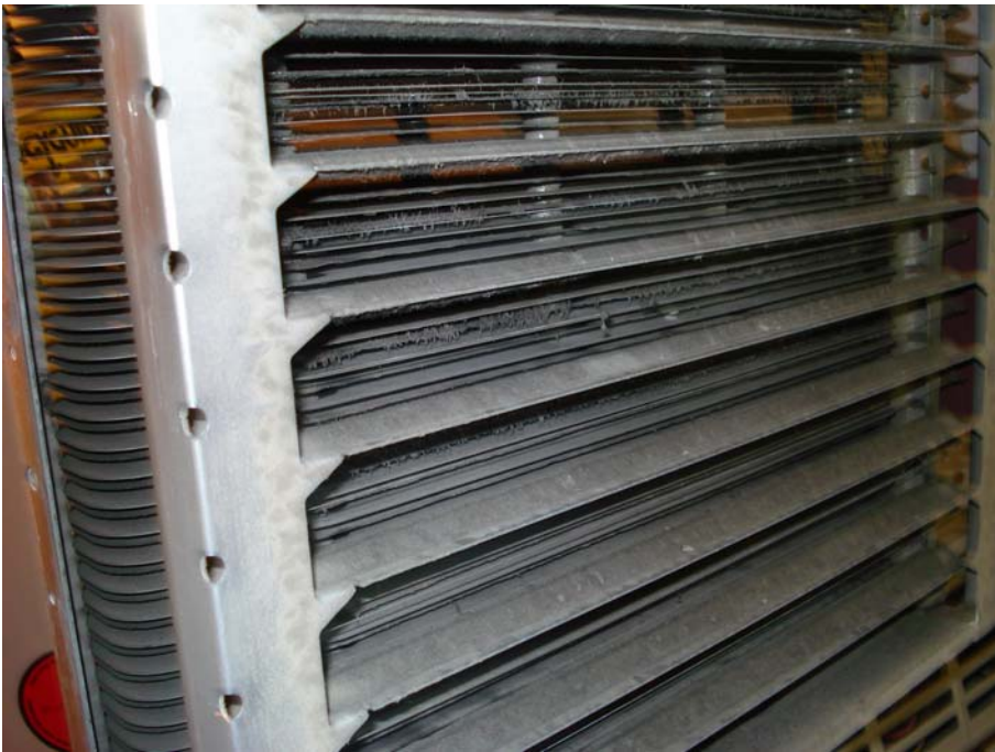
Dirty electrostatic filter close-up.
