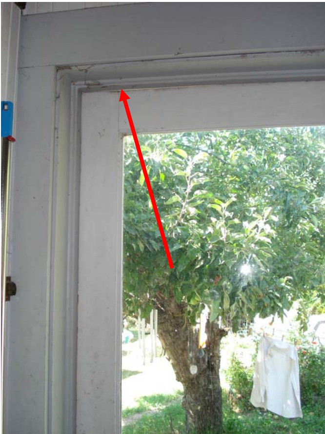
Back door doesn't seal well. Large gap at upper left corner
