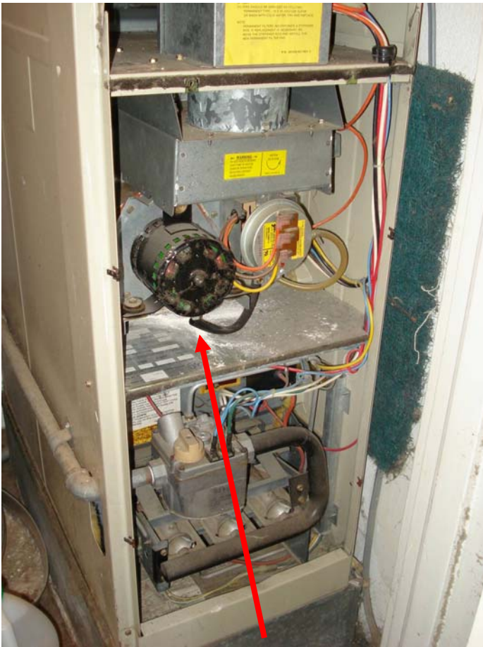
White powder below motor appears to be some type of corrosion indicating possible excessive moisture.
