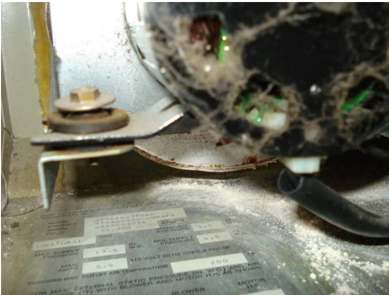
Close up of the same corrosion.
