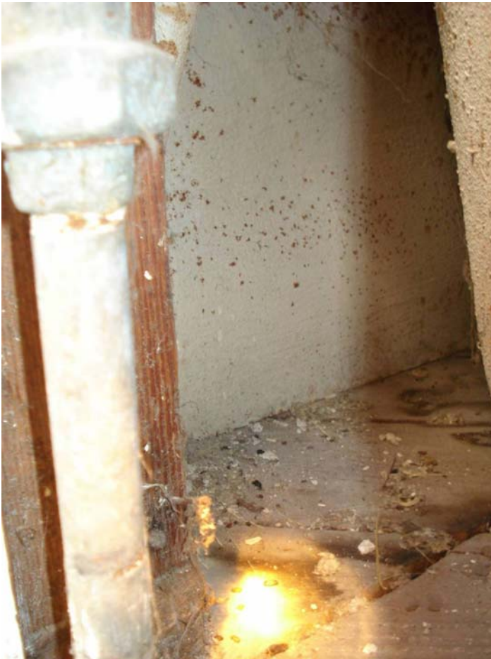
Wall behind tub from exterior. Some rodent droppings found.
