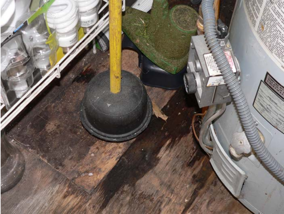
Water under and behind water heater in cottage. Probable leaking water heater.
