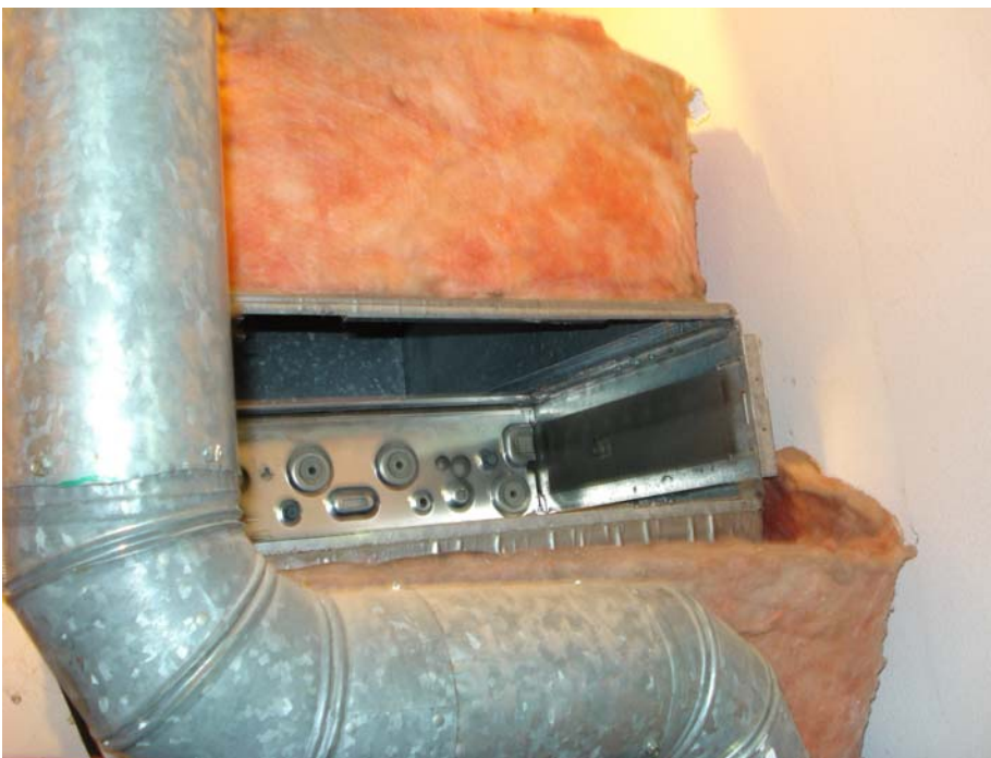
Electrostatic cleaner in furnace. The filter was dirty.
