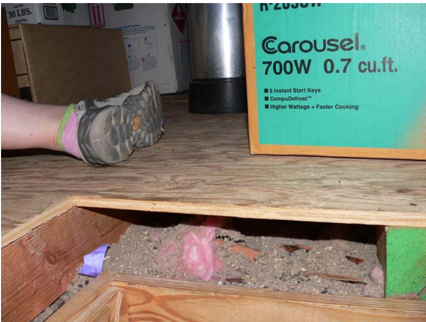
Insulation in the attic is only about 3" thick.
